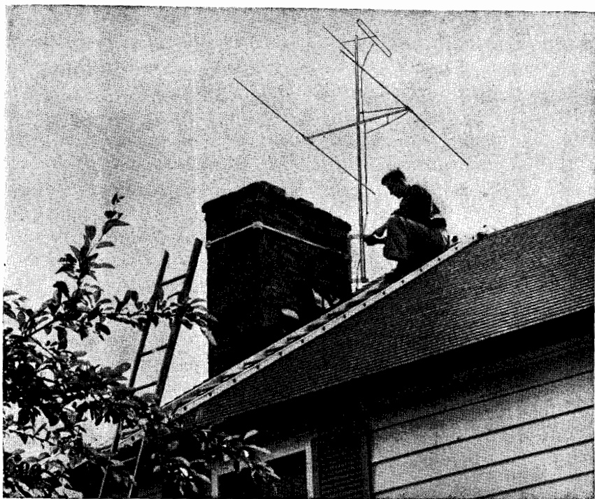
Fig. 5. Use of double-extension ladder and single ladder with roof hooks to get up to the chimney of a house safely for installing a television antenna. (RCA Victor photo)
