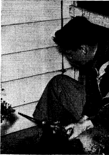
Fig. 10. Drilling a hole through the wall of a house into the basement for bringing in the television transmission line. (RCA Victor photo)
