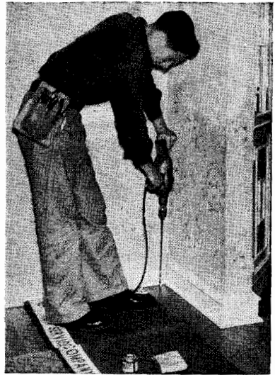
Fig. 11. Drilling a hole in the floor close to the wall behind the selected receiver location, for bringing up the transmission line from the basement. (RCA Victor photo)
